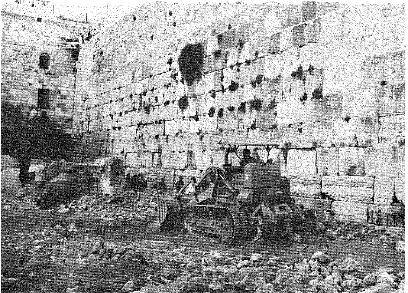
Clearing rubble from the Kosel Ma'aravi site after it was taken by Israeli forces.
